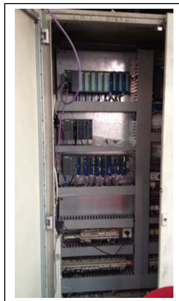
CABINET WITH SIEMENS S7-300 PLC
