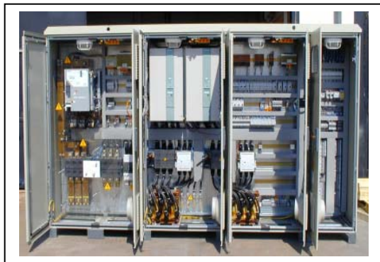
SIEMENS INVERTER CABINET FOR CRANE TRANSLATION
