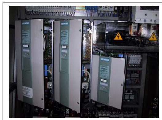
INVERTER CABINET MOTORS SYNCHRONIZATION
