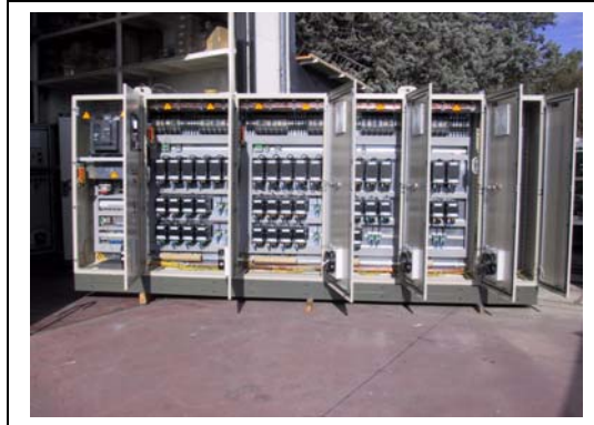
POWER CABINET FOR HEATING FURNACE GLASS PRODUCTION
