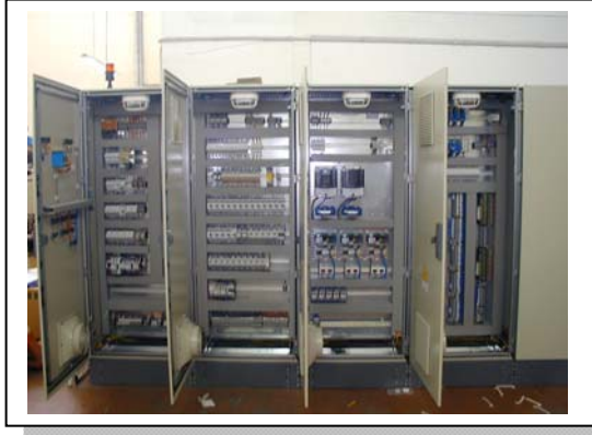
ROCKWELL PLC CABINET FOR "BATCH PLANT" PLANT
