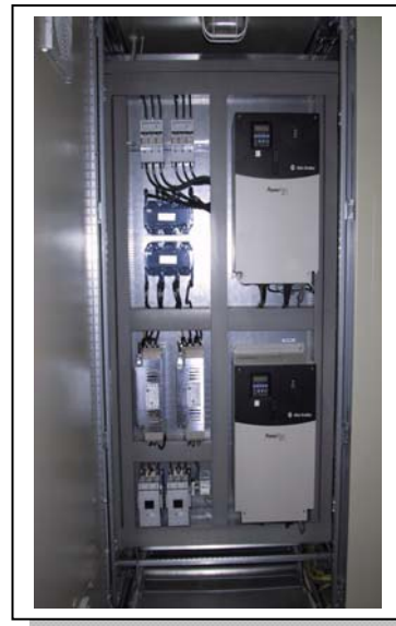
INVERTER CABINET CONVEYORS SPEED MANAGEMENT
