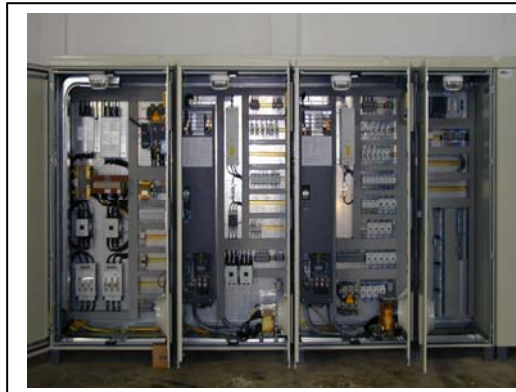
1200 A DRIVER CABINET FOR CRANE HOIST
